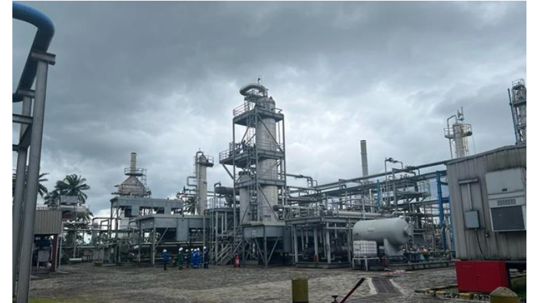
Modular Refinery Train 3 at 5000 bbls/d capacity
