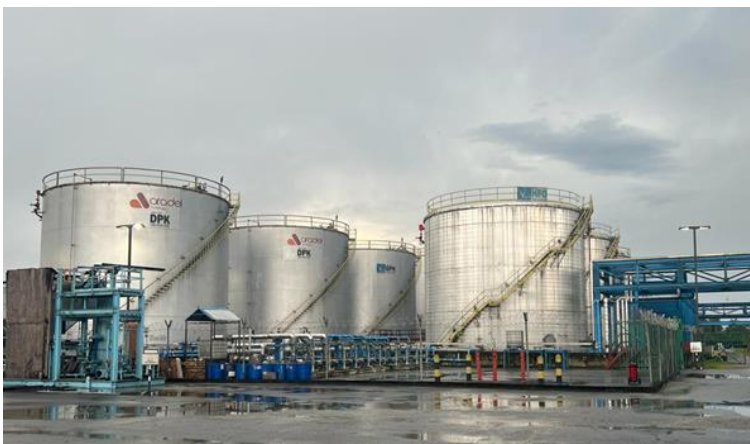
Product Storage Tanks for PMS, Naphtha, DPK, AGO, MDO & HFO
