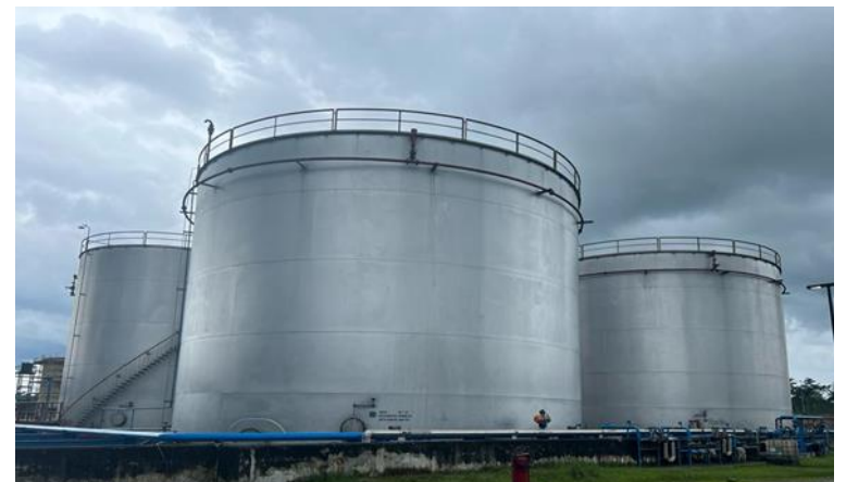
Two 20,000 bbls Crude feed and One 10,000 bbls Naphtha Storage Tanks
