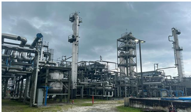
Pre-Commissioning of 3000 bbls/d capacity PMS & Naphtha Trains
